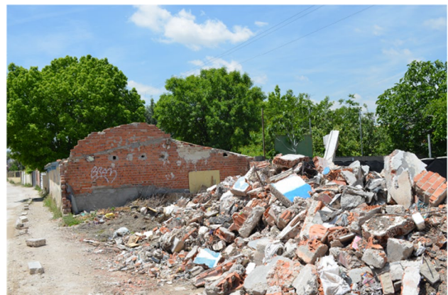
Fig. 2 Rubble from a home destroyed by city officials in Spain
